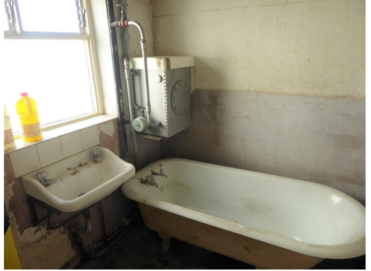
Wash hand basin, high level w.c, freestanding bath.
